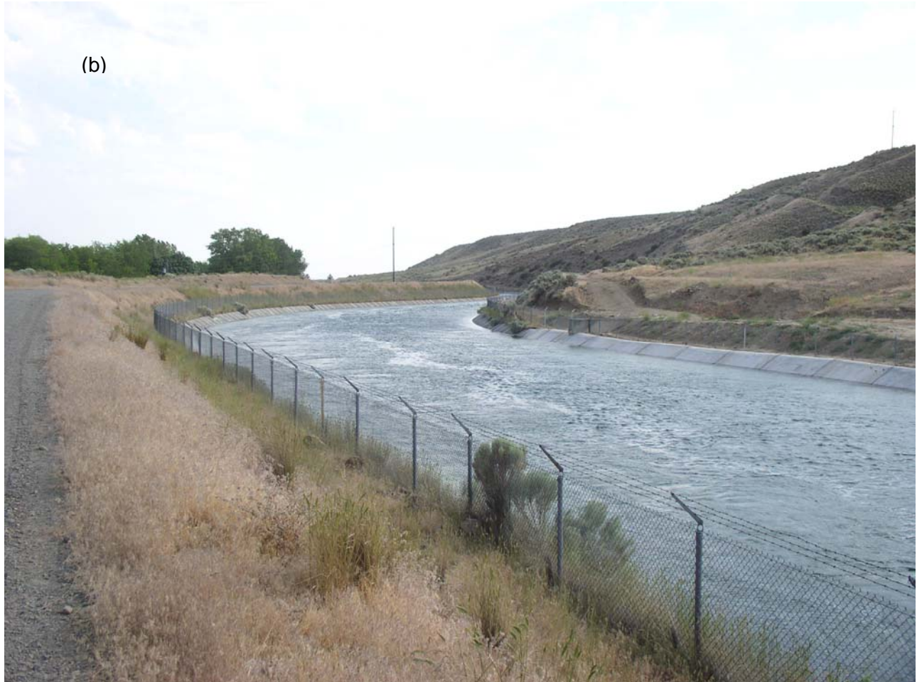
Section of the 50 year-old canal of the Quincy-Columbia Basin Irrigation District, Washington State, USA repaired in 2003 with composite Ethylene-Vinyl Acetate (EVA) liner (0.5 mm) between two non-woven geotextiles. The composite liner was covered with 75 mm poured concrete. Side slopes are 1.5H: 1V. Photos taken of the same section during repair (a) and when the canal back in service (b) [Photo courtesy: Huesker Inc.]
